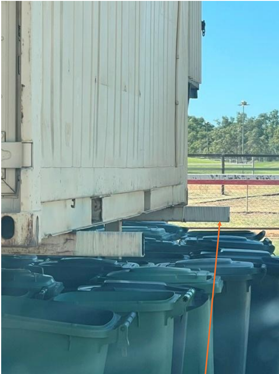
Racecourse. Horizontal steel frame at head height.
