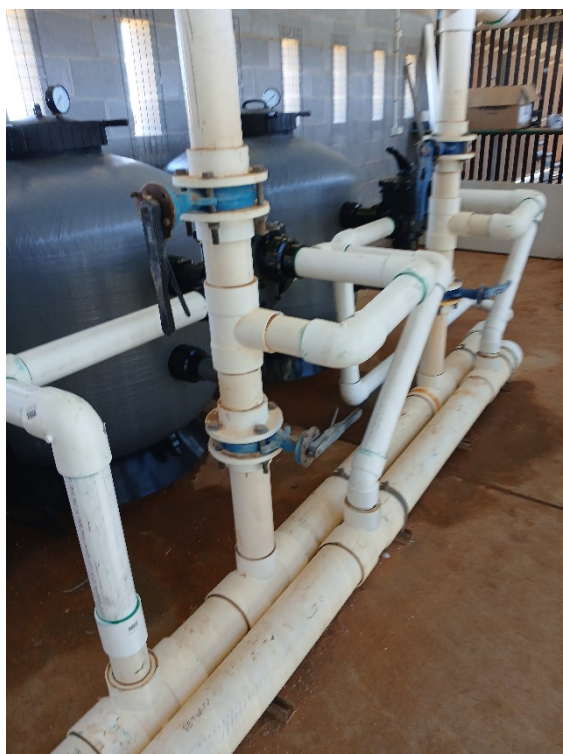
New filters and plumbing
